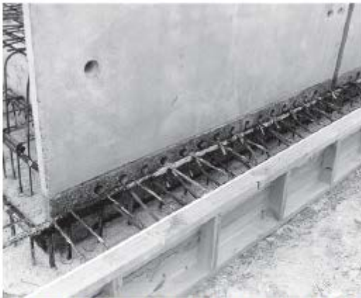
Figure 4.14: Connection between base of wall panel and foundation (Rotorua District Council Civic Centre)
